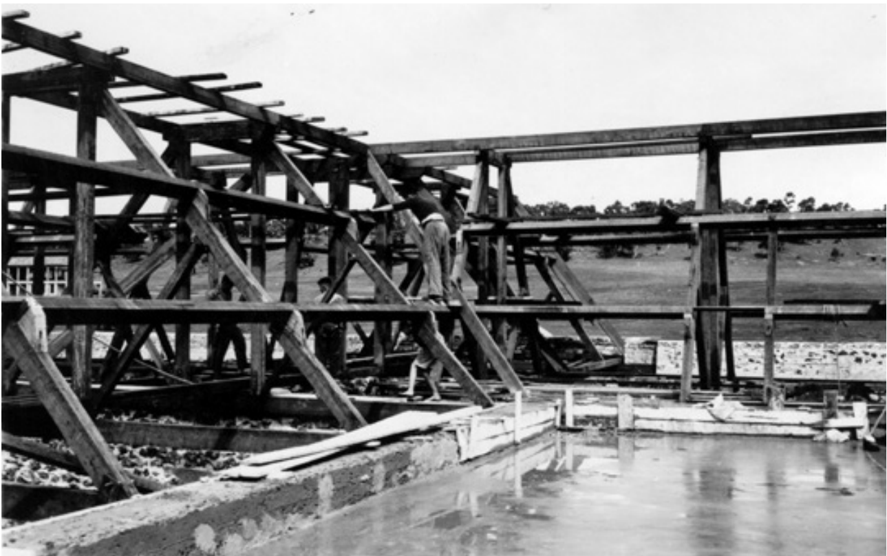
Bindoon Boys’ Town, building work, 1952. Photograph from Western Australia Government photographer collection. Source: State Library of Western Australia .
