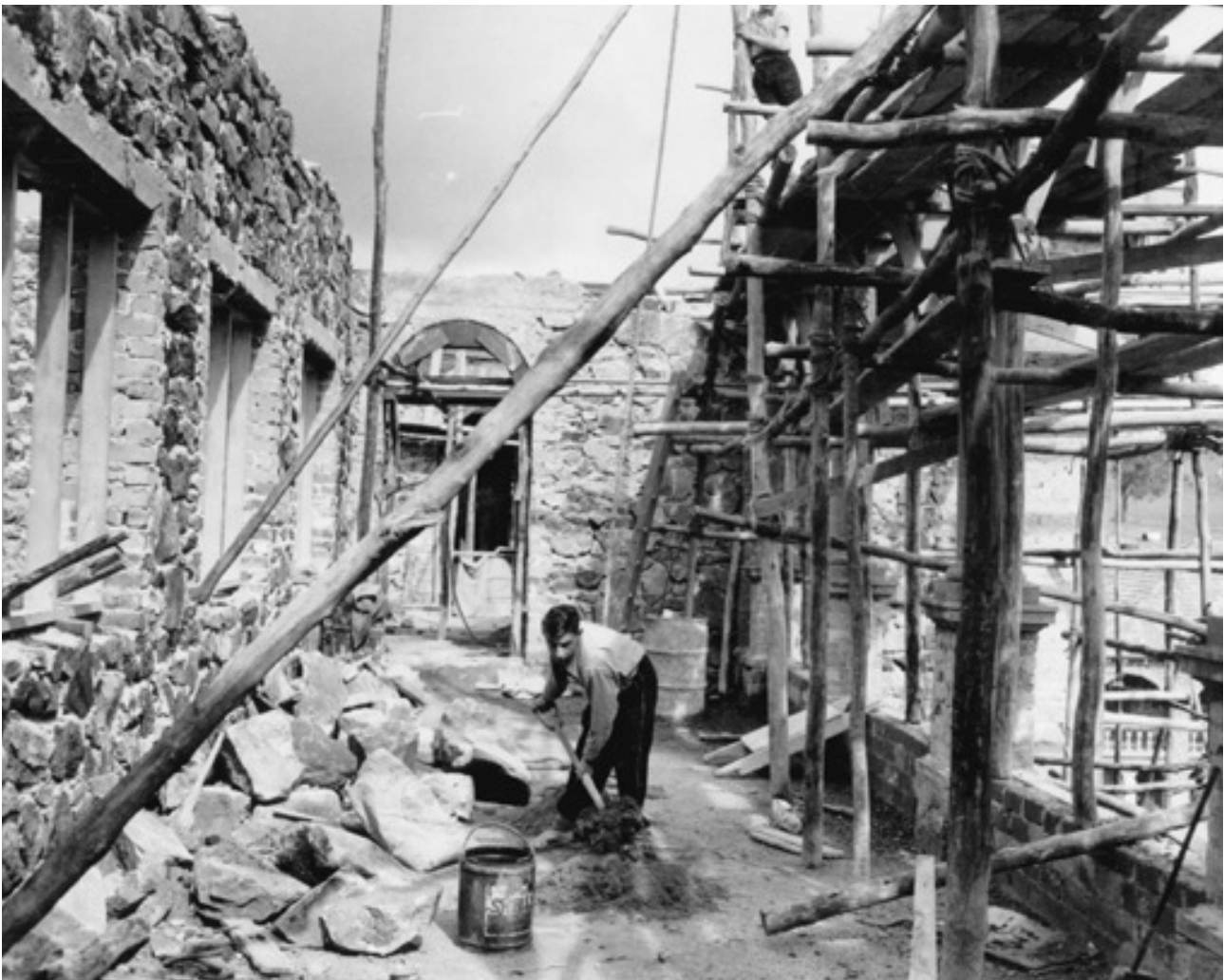
Bindoon Boys' Town, construction of administration building, 1952. Photograph from the Western Australia Government photographer collection. Source: State Library of Western Australia .
